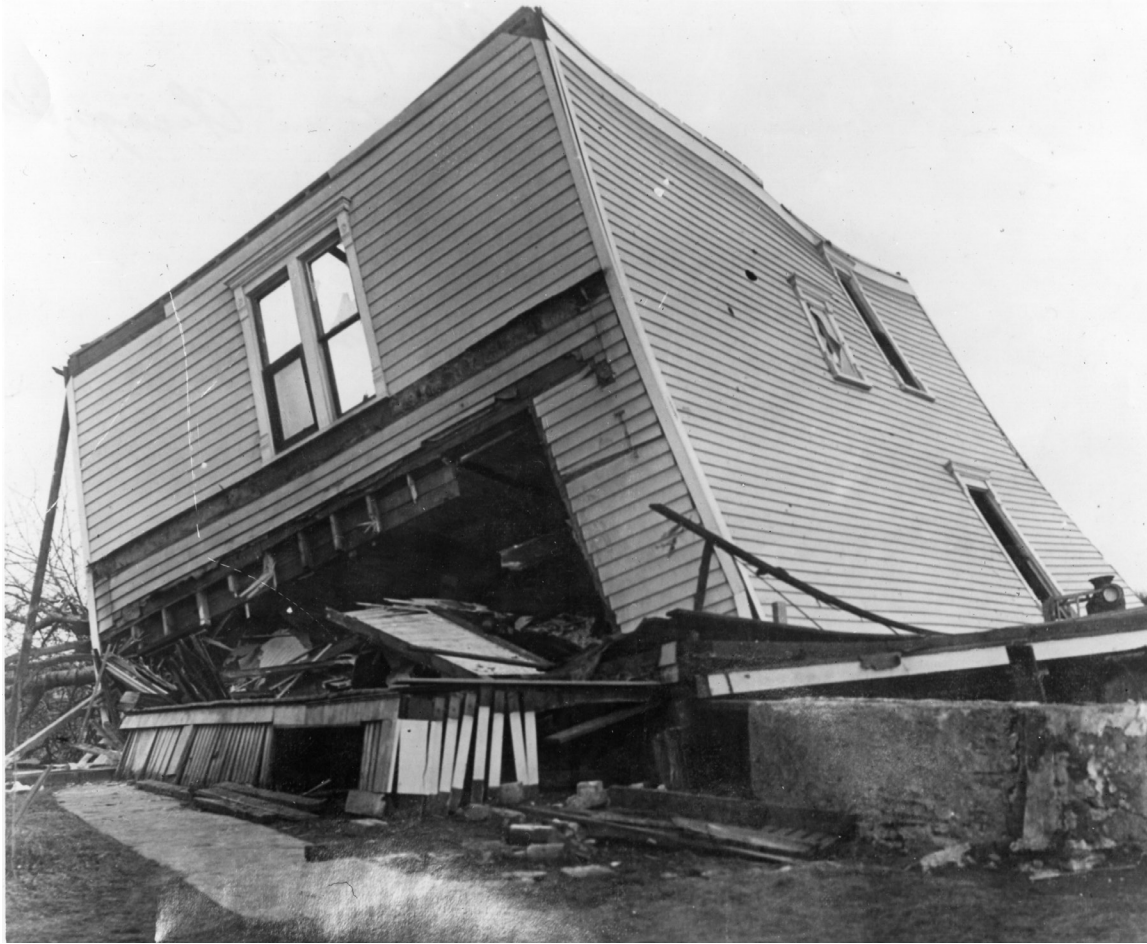
A Dunning neighborhood storefront slid off its foundation during the storm.
