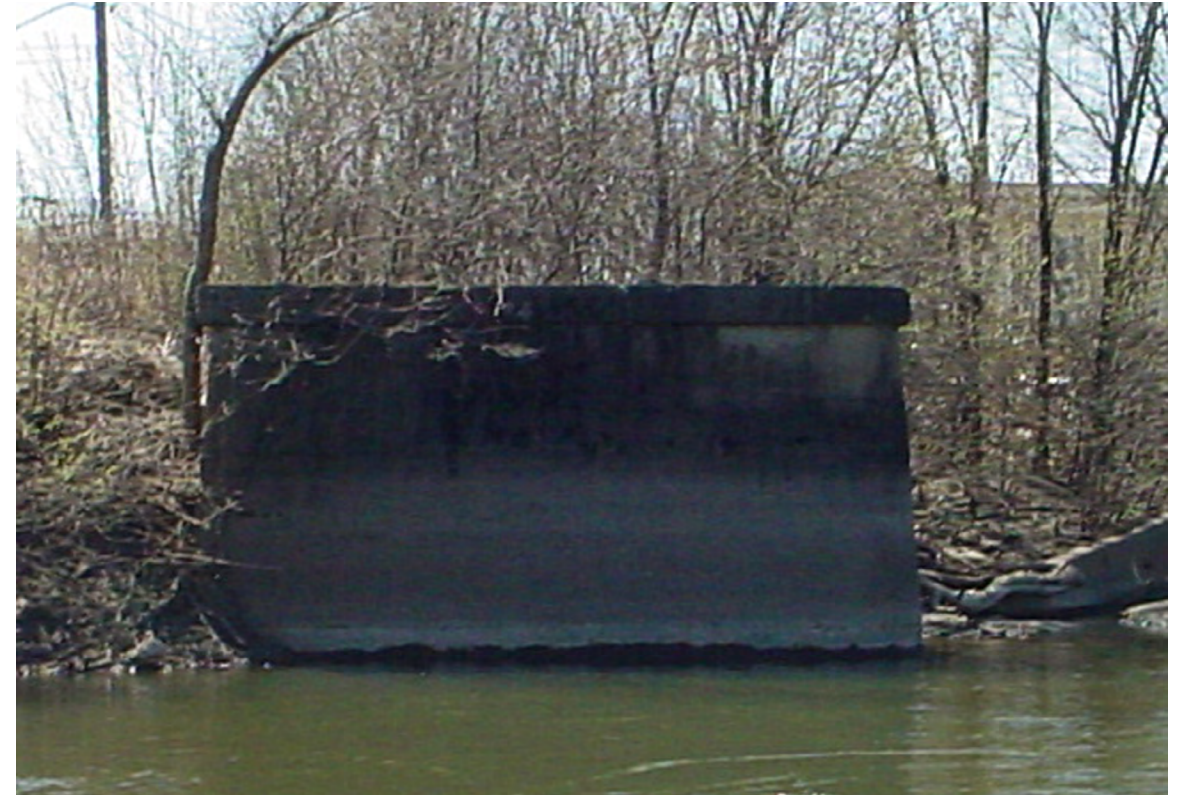
Two concrete pylons on each side of the Des Plaines River just south of the Belmont Avenue bridge once supported the Chicago Terminal Transfer Railroad Company's train trestle. 12. Photo by Frank Suerth
